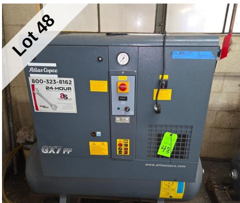
2016 ATLAS COPCO 10-HP ROTARY SCREW AIR COMPRESSOR
